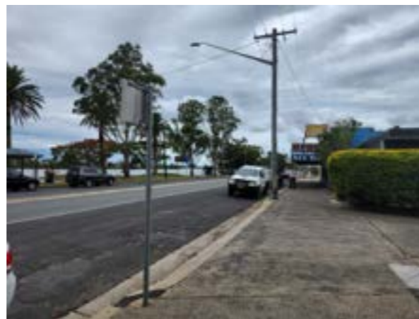
Existing pavement conditions-crossover at Motel
