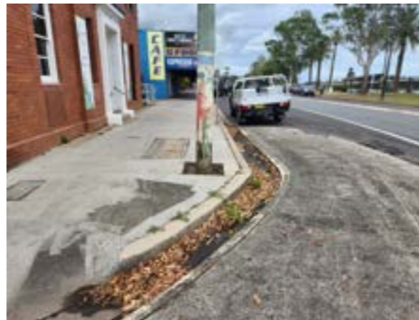
Existing pedestrian pavement conditions-corner of Duke Street to Seafood Takeaway
